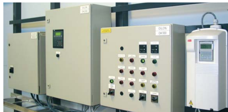
All-inclusive burner automatics: oxygen (O 2 )/pressure difference/cascade control
